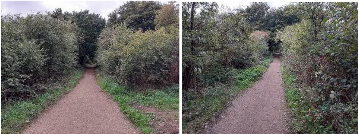
Figure 7. Vegetation encroaching on width of surfaced path.
