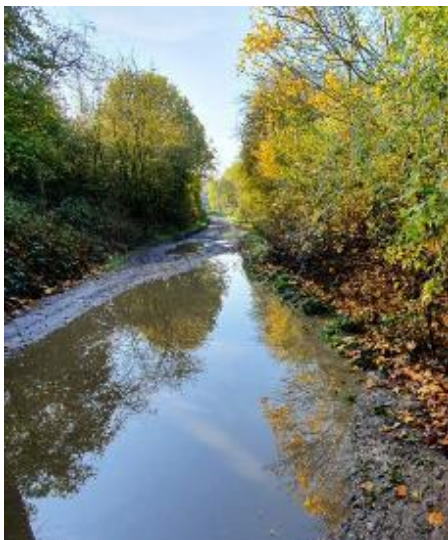
Figure 4 Flooded surface by B653 underpass
